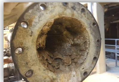
Struvite buildup in sludge piping system
